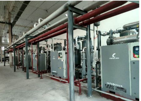
Project Client Pharmaceutical & Food Industry Machine Model 10 × 45 m³/min Energy-Efficient Refrigerated Air Dryers + Blower-Heated Regenerative Adsorption Dryers
