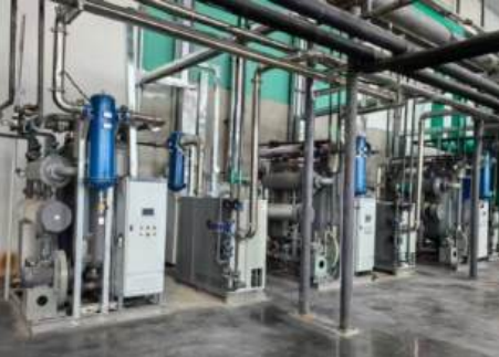
Project Client New Energy Materials Machine Model 2 Zero-Air-Loss Blower-Heated Regenerative Adsorption Dryers + 3 Refrigerated Air Dryers + 350 m³/h Nitrogen Generator
