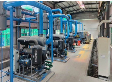
Project Client Petrochemical Industry Machine Model 8 × 250 m³/min WH Series Refrigerated Air Dryers
